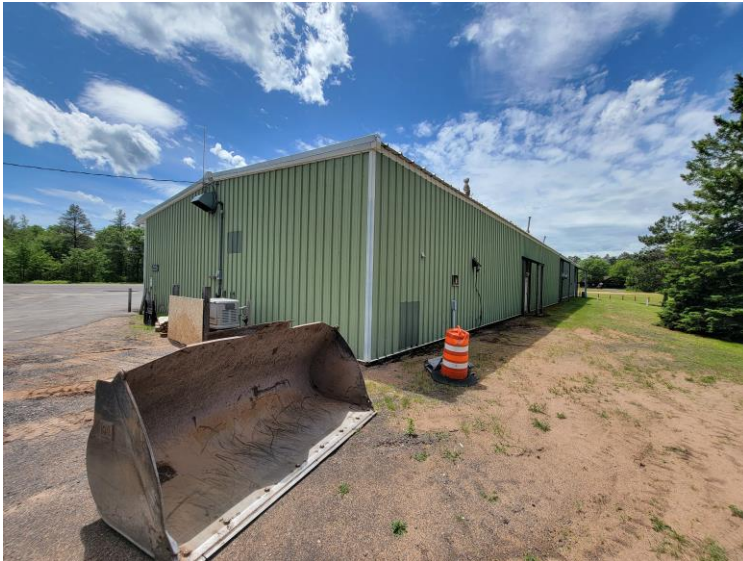
NE View, Lack of Proper Storage
